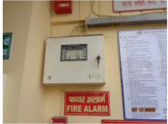
06. Fire alarm control Panel.JPG
